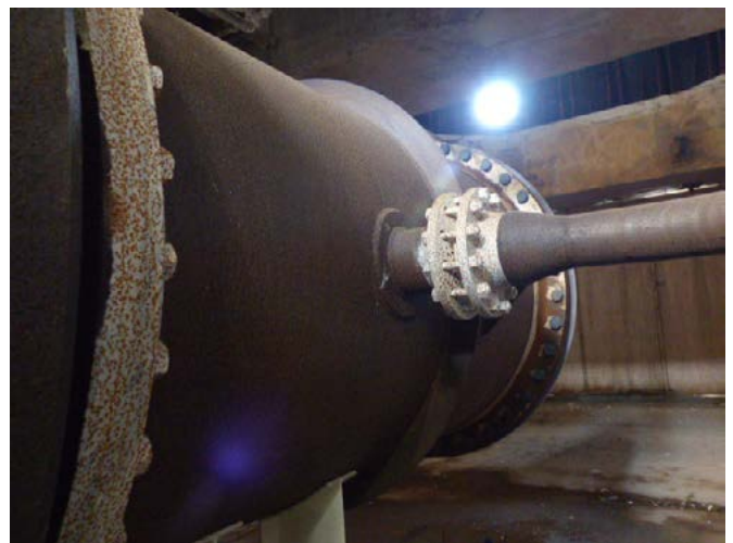
Figure 3: Large section of pipe with asbestos-containing insulation residues
