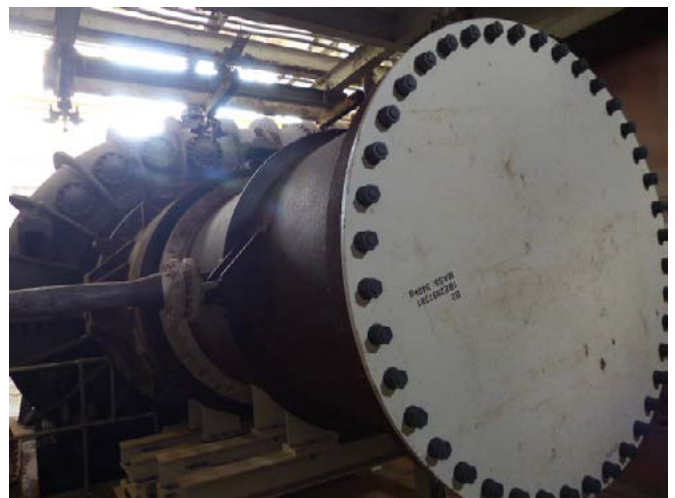
Figure 2: Large section of pipe with asbestos-containing insulation residues
